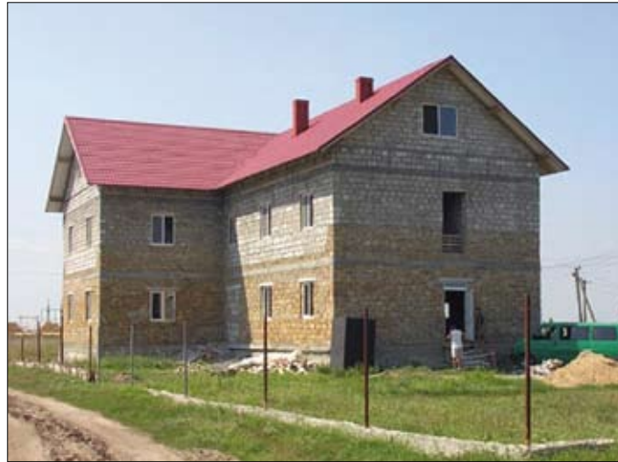
Construction of Seminary and Mission Centre in Ukraine – Current project supported since 2003
