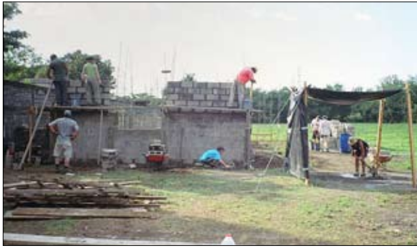
Hands-on mission in Chinandega, Nicaragua, December 2006. Workers from Faith, Grand Prairie, Good Shepherd, Valleyview and Redeemer, High Prairie worked on two dormitories. $23,000 was raised by the above congregations and St. John's, Wembley to fund the construction.
